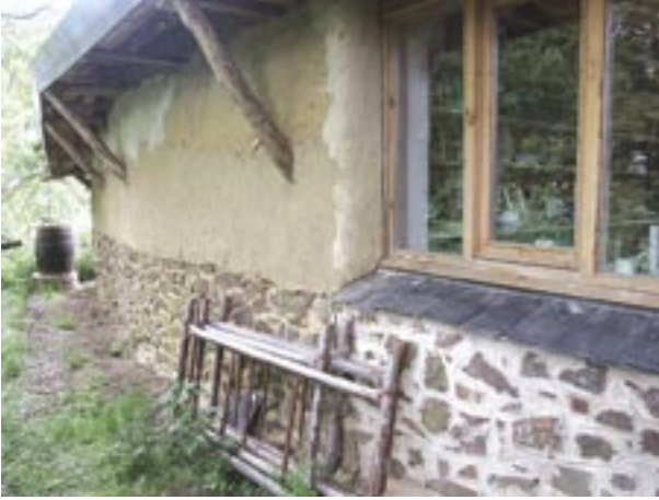
This shows the gridshell building from the previous page but from the outside, with stone walls using both lime and clay mortars, and clay external render under a large roof overhang.
